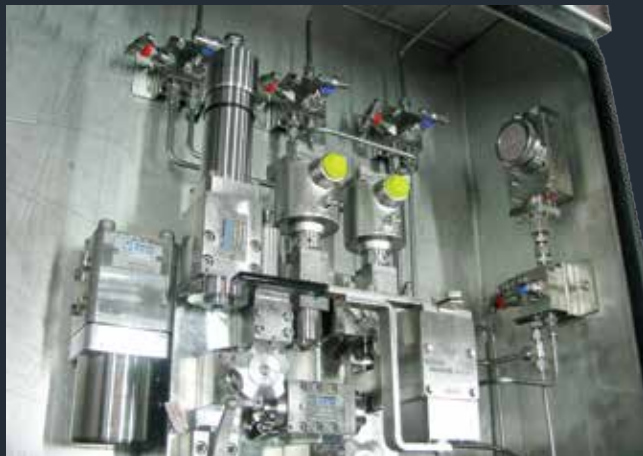
CONTROL CABINET (Project VEGA PLEYADE - Total - Argentina)
