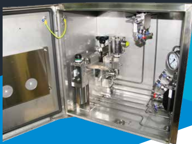
CONTROL CABINET (Project BP QUAD 204 - BP - United Kingdom)
